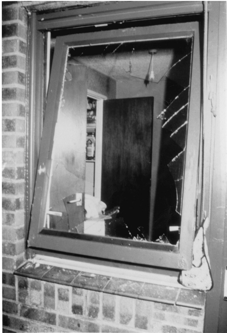
Fig. 3. Broken kitchen window as viewed from outside.
